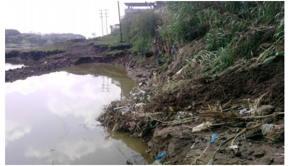
चित्र.6- Bank erosion at Ordinance factory, Kirki, Pune
